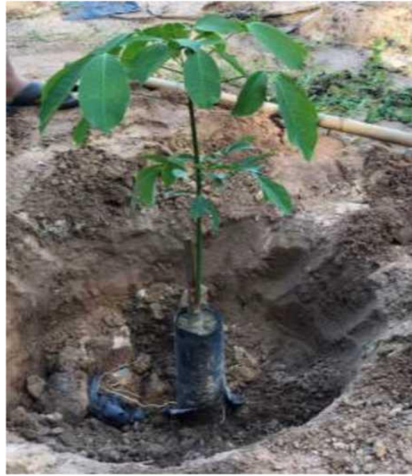
Figures IV.1b. Placing the bag into the hole and cutting the PE bag
